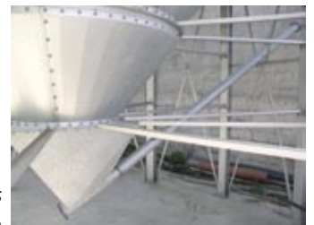
Solid attachment of legs in the silo.
